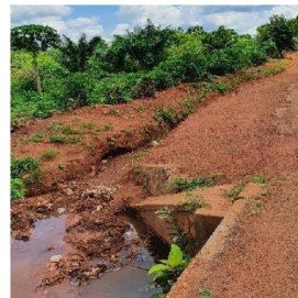
Photos 48: Absence de drainage
