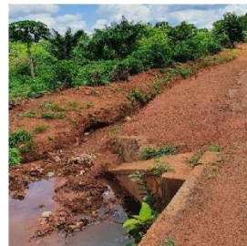
Photos 48: Absence de drainage
